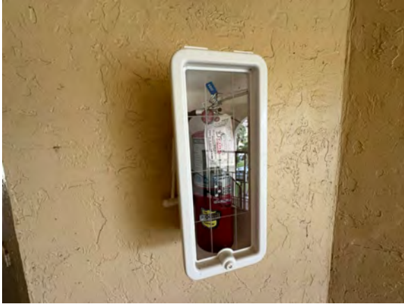
VIEW OF TYPICAL FIRE EXTINGUISHER
